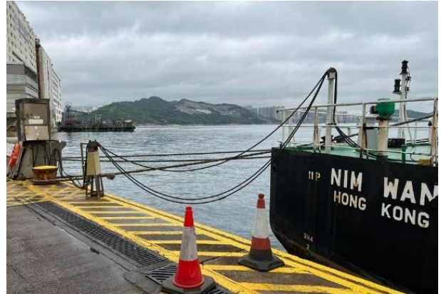
Shore power station at IETS
